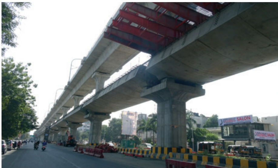
The new metro line in the Indian metropolis of Nagpur is being built with support from German ODA via KfW Development Bank.
