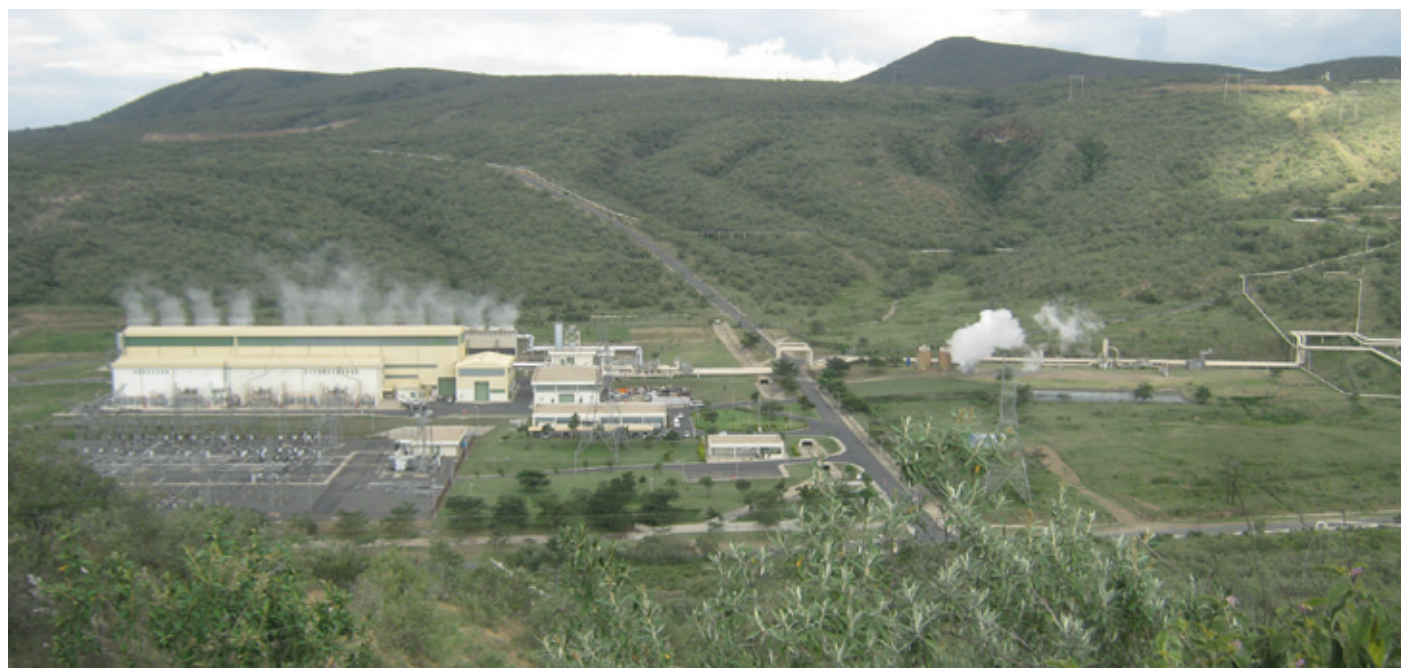
Geothermal power station in Kenya.
