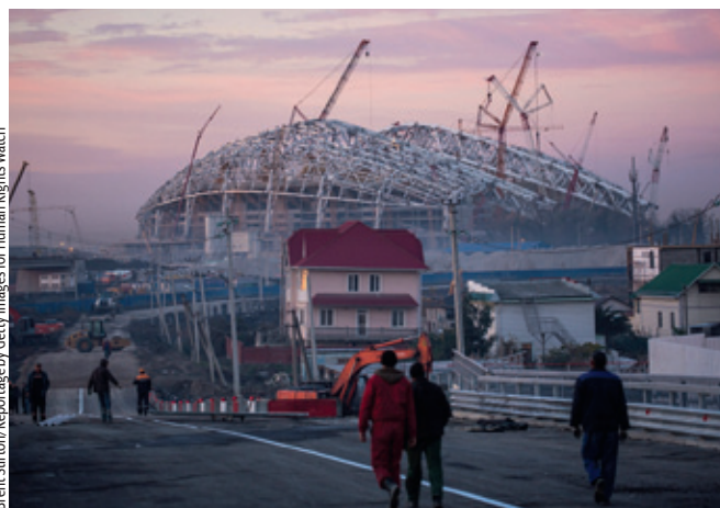
Labour migrants on their way to the building site of the Olympic stadium in 2012.
